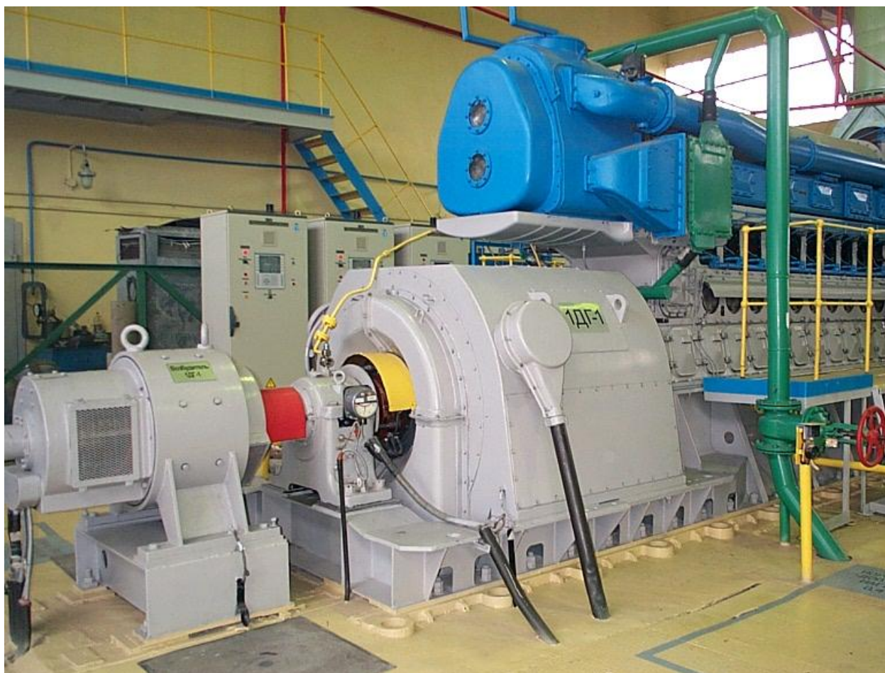
Figure 4 - An emergency Diesel generator (foreground) and associated control system (background). In nuclear power plants such systems typically are used to provide backup electrical power necessary to execute vital safety functions, including core cooling, in event of loss of the offsite power that normally serves. (Photograph courtesy of Diakont Advanced Technologies)Safeguards
