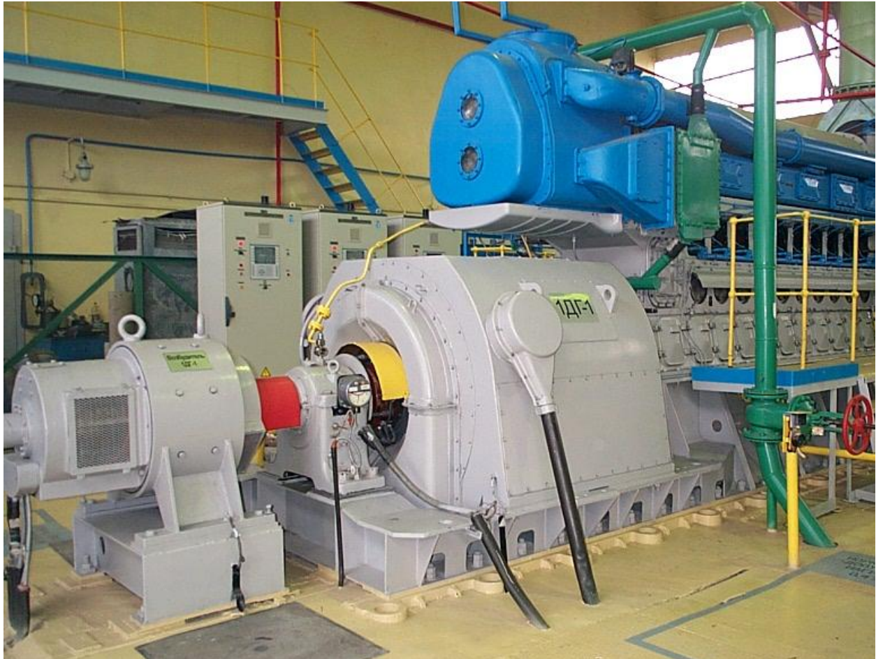
Figure 4 - An emergency Diesel generator (foreground) and associated control system (background). In nuclear power plants such systems typically are used to provide backup electrical power necessary to execute vital safety functions, including core cooling, in event of loss of the offsite power that normally serves. (Photograph courtesy of Diakont Advanced Technologies)Safeguards
